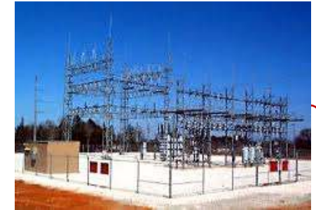
Substations (step down)
