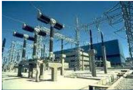
Substation (step up)
